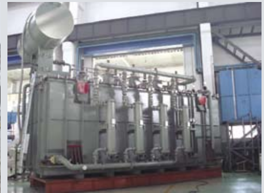
The first main transformer (300 MVA/220 kV OFWF) positioned in the substation of 2010 Shanghai Expo -- the largest underground substation in Asia
