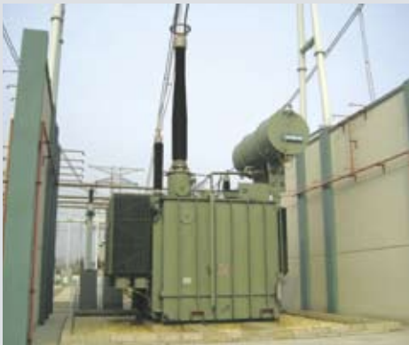
334 MVA/500 kV transformer (AF) for Jiangnan substation in Yichang, Hubei
