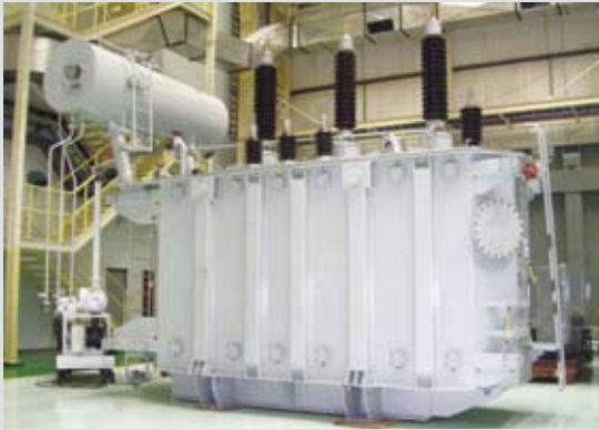
50 MVA/110 kV transformers for Beijing Olympics Aquatic Park & Wukesong Basketball Indoor Stadium
