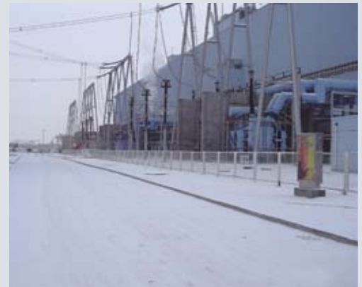
63 MVA/220 kV transformer (ONAN) for Datang Tuoketuo substation in Inner Mongolia
