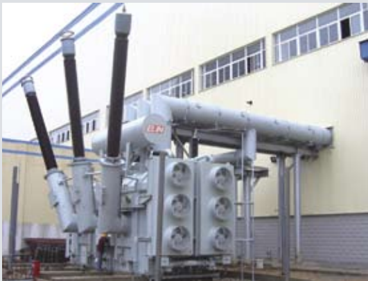
370 MVA/500 kV GSU transformers for Henan Datang Luoyang thermal power generation expansion scheme
