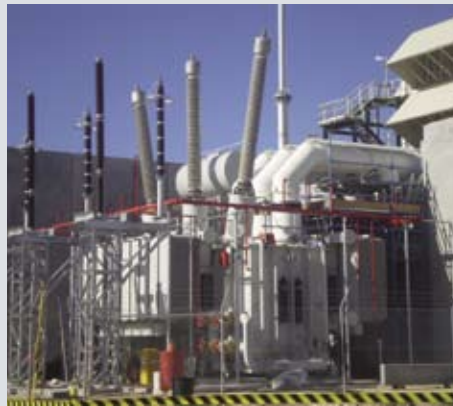
Two units of 225 MVA/330 kV GSU transformer for AUS809 Neerabup gas-fired station in Australia
